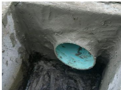
Example of a BAD pipe installation. Protruding past the internal wall of the structure, poor grouting, and wrong position.
