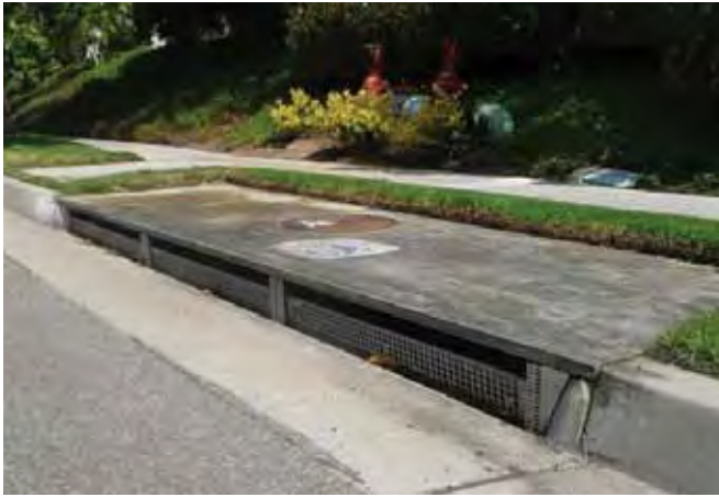
FIG. 6. Curb grate installed at a catch basin opening in the drainage area.
