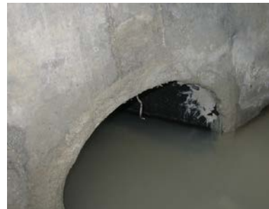
Example of a GOOD pipe installation. Pipe flush with the internal wall of the structure, clean grouting, and proper position.
